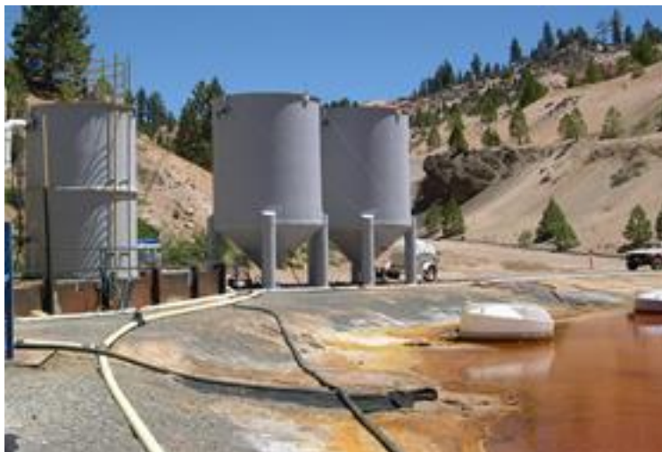
Figure 1-5: Silos can be used to raise the pH of AMD by actively dosing it with alkaline chemicals. ( http://www.epa.gov/nrmrl/lrpcd/etsc/basic.html , accessed 10/30/2013).
