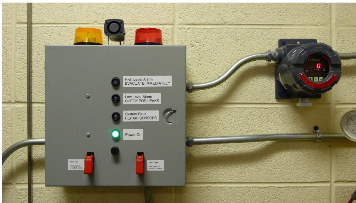
Figure 2.20: Gas detection system control box and NH 3 sensor control unit showing NH 3 concentration in ppm. Visible on the control box are the status indicator LEDs, on/off and alarm test switches, amber and red strobe lights, and siren. Not pictured are the NH 3 , NO, and NO 2 sensors and the NO/NO 2 control unit.
