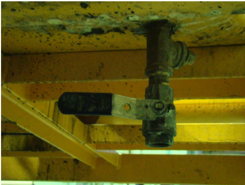
A6. Bottom Drain Valve
