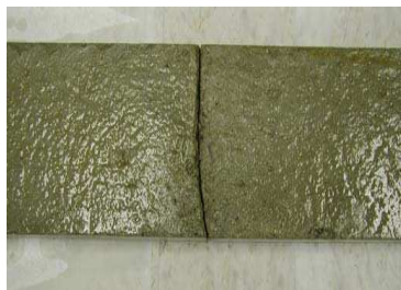
Concrete Slab with Defect – Crack
