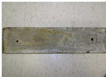
Concrete Slab with Defect - Hole
