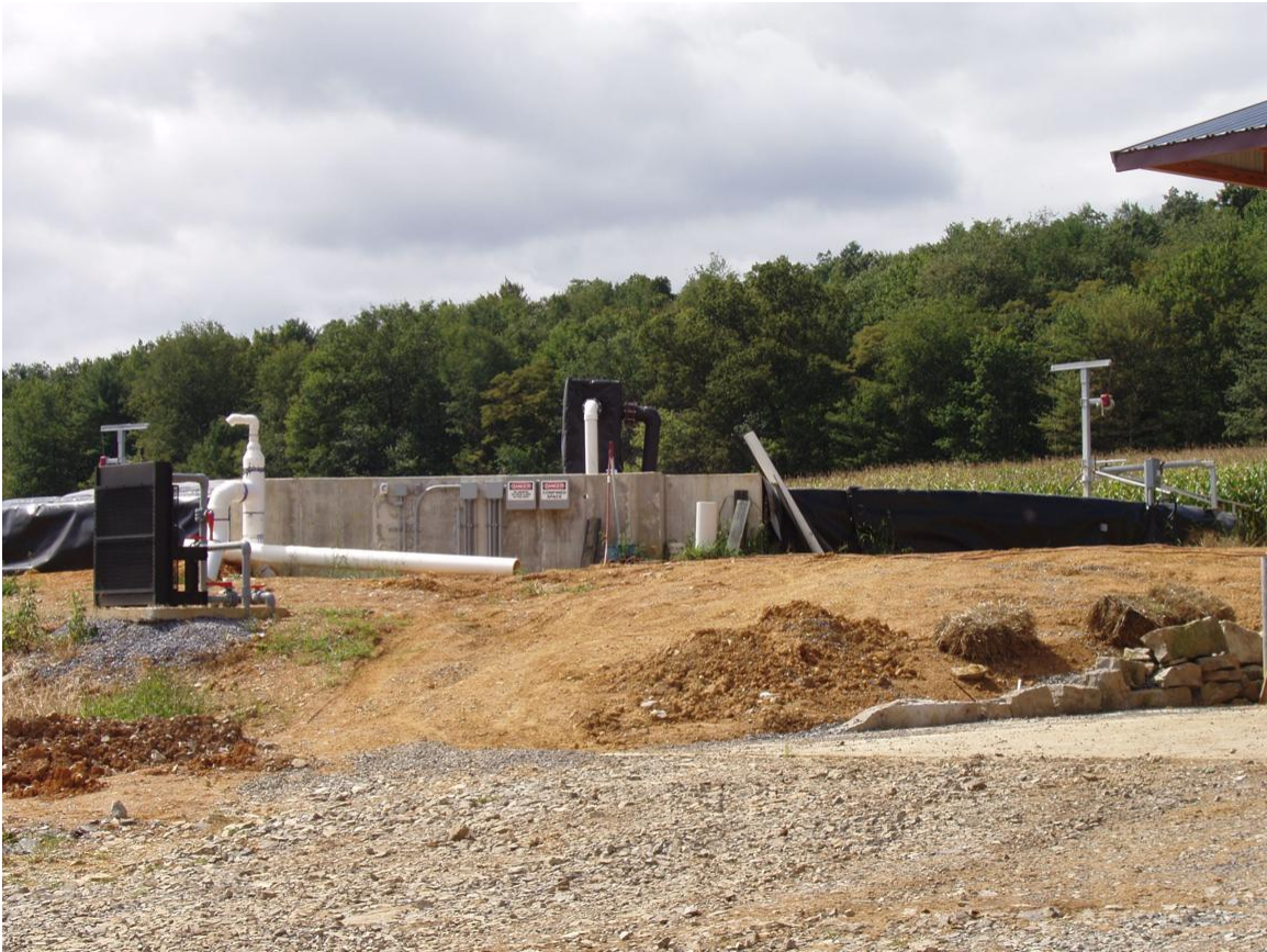
Figure 6.18: Penn England Digester
