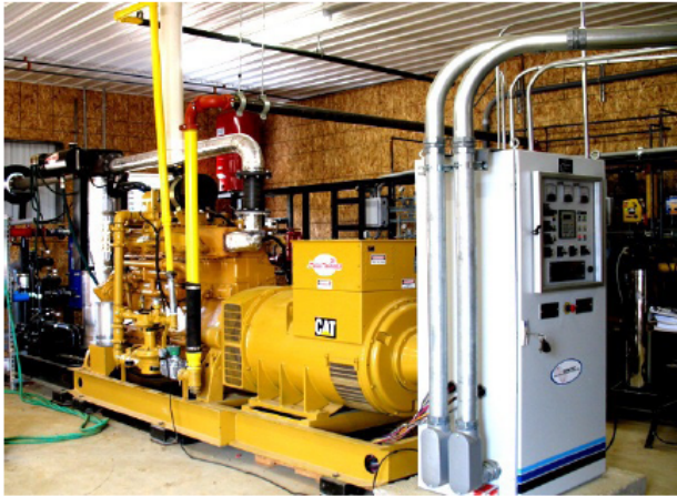
Combined Heat and Power Unit (CHP)
