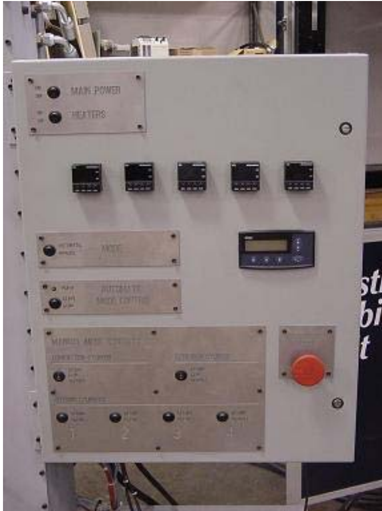
Figure 30: Outside of Control Box
