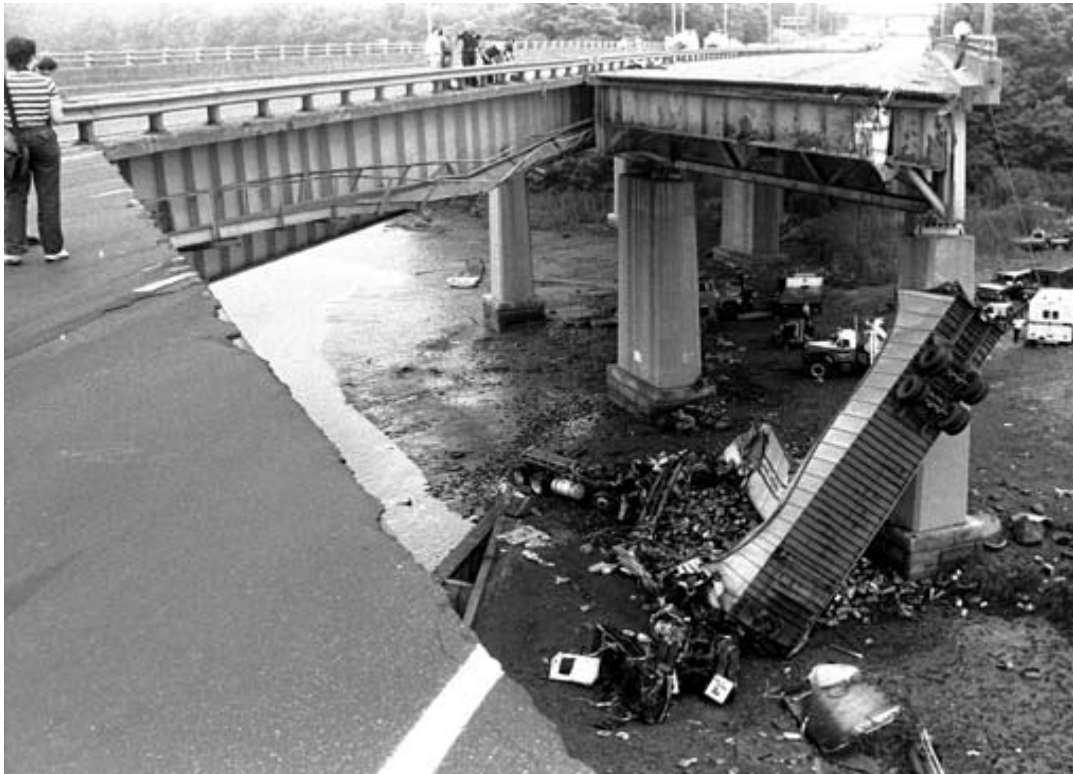
Figure 2-3. Mianus River Bridge Collapse
