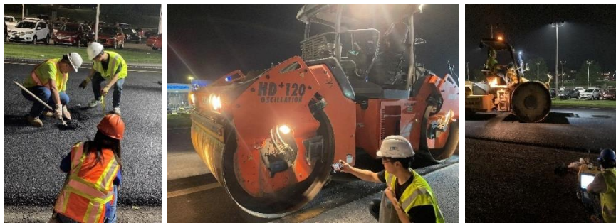
Figure 4-4 SmartKli ® installation and data collection in the Altoona project
