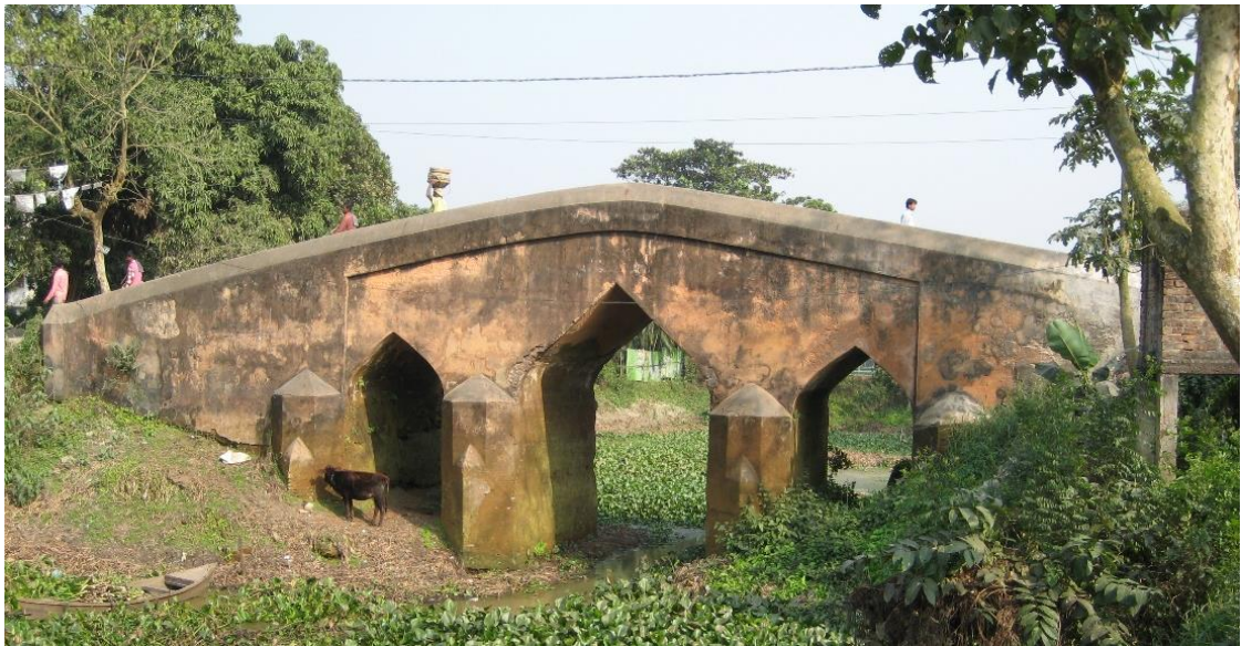
Figure 16: The Mughal Bridge (Pool) on the Pankhiraj River at Panam Nagar, (Source – Author, 2020)
