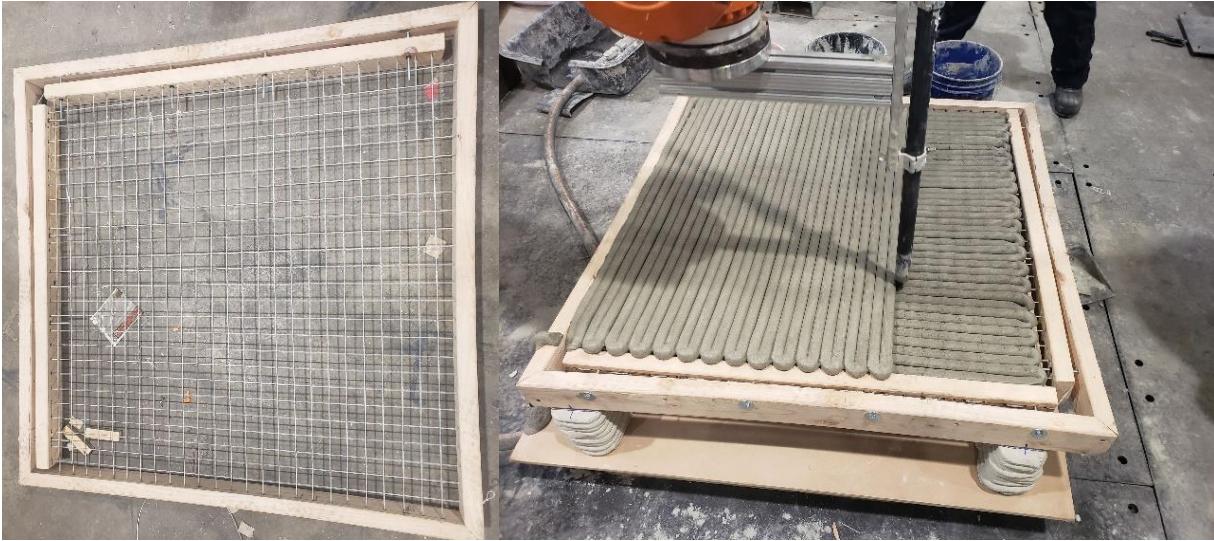
Figure 5-4: Variable tension 1×1 meter mesh as built on left and on second layer on the right.
