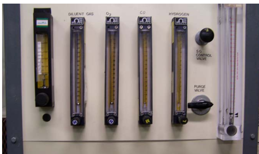
Figure 3.5: A photograph of the control panel used in this project. It should be noted that the panel was adapted from a previous project leaving several meters unused.
