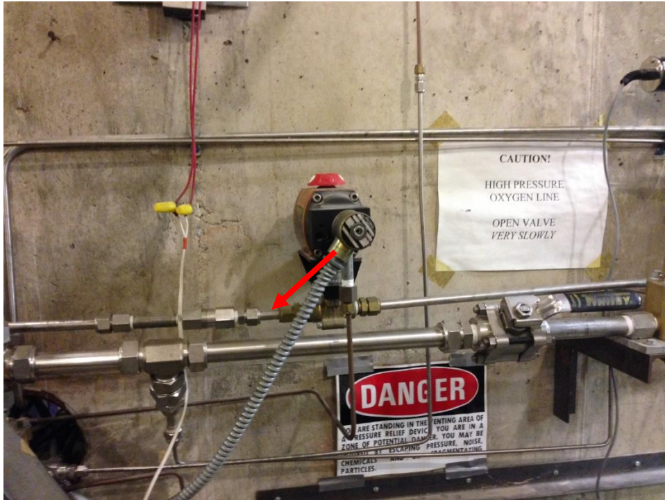
Nitrogen Purge Valve (RM 128)
