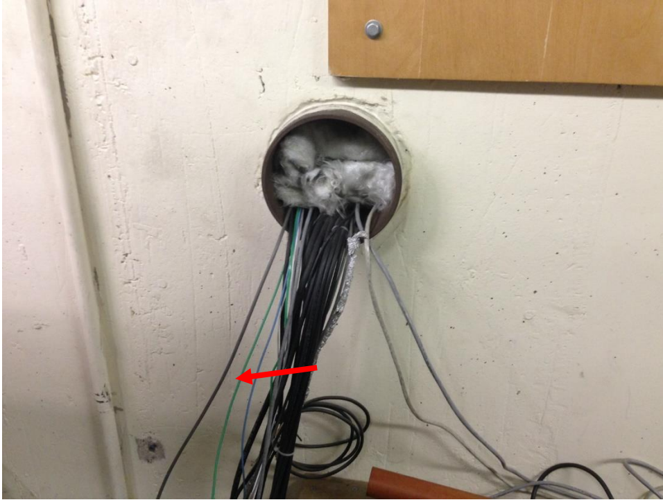
BNC and Igniter Wire Feedthrough to Control Room (Control Room)
