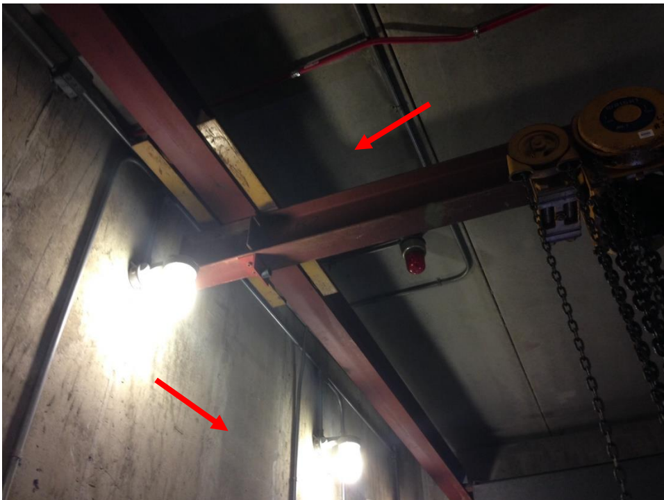
Relay Wires (RM 127)
