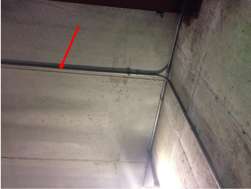
Relay Wires (RM 127)
