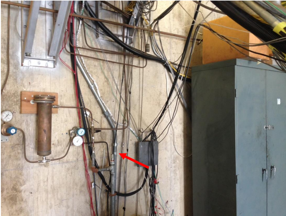
BNC and Igniter Wire Feedthrough to Control Room (RM 127)
